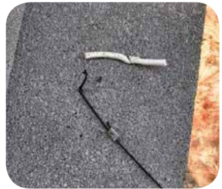
A vinyl coated, stainless steel tie cinched so tight that it cut through the wire. Photo source: PV Pros, Inc.
